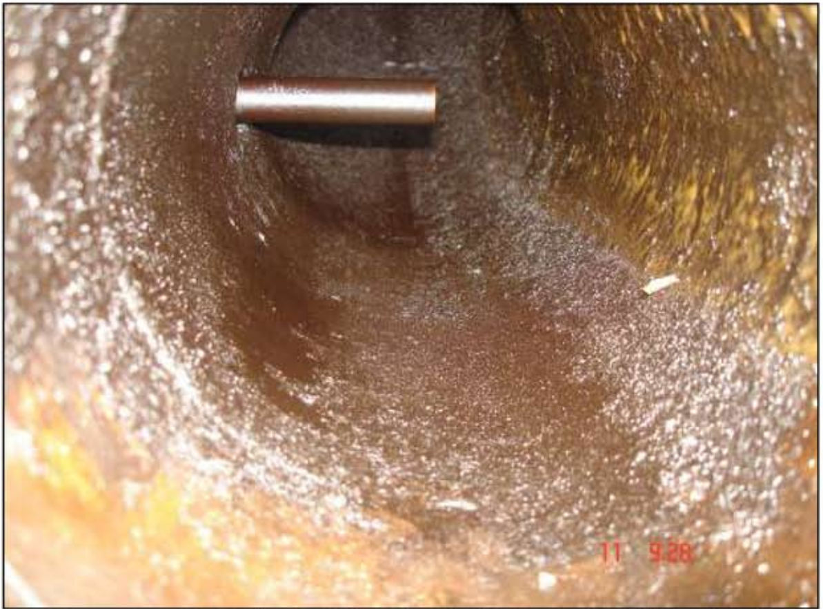
Figure A – EXTREME CONDITION OF PIPING IN SOME MACHINES
